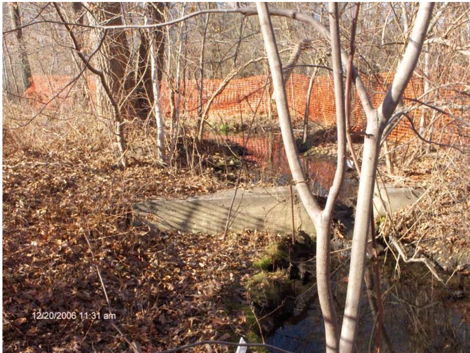
SCENE: View of the concrete weir at the terminus of the drainage swale. Photograph taken facing south.
