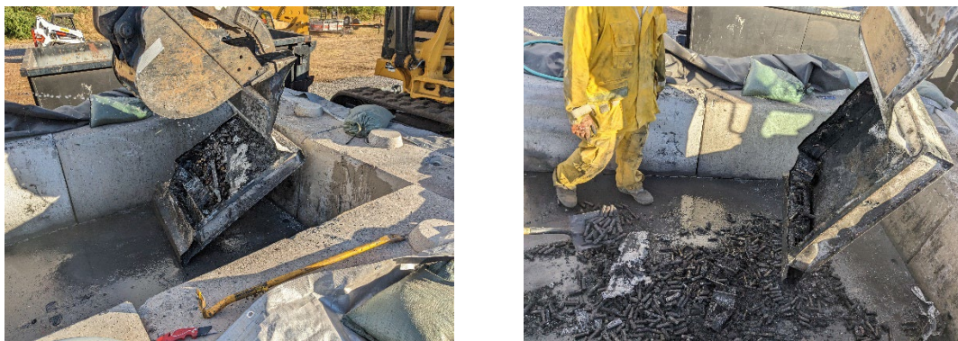
Figure 12. An excavator with thumb peels open a BESS/ESS system revealing the cylindrical cells inside, water is applied to suppress dust at the 2023 Maui Wildfire Response.
