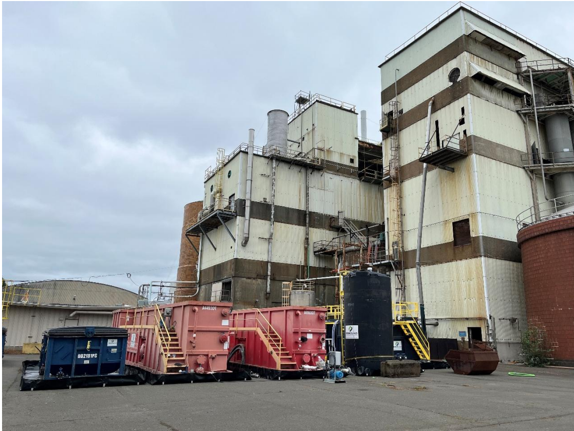
Treatment plant equipment set-up.
