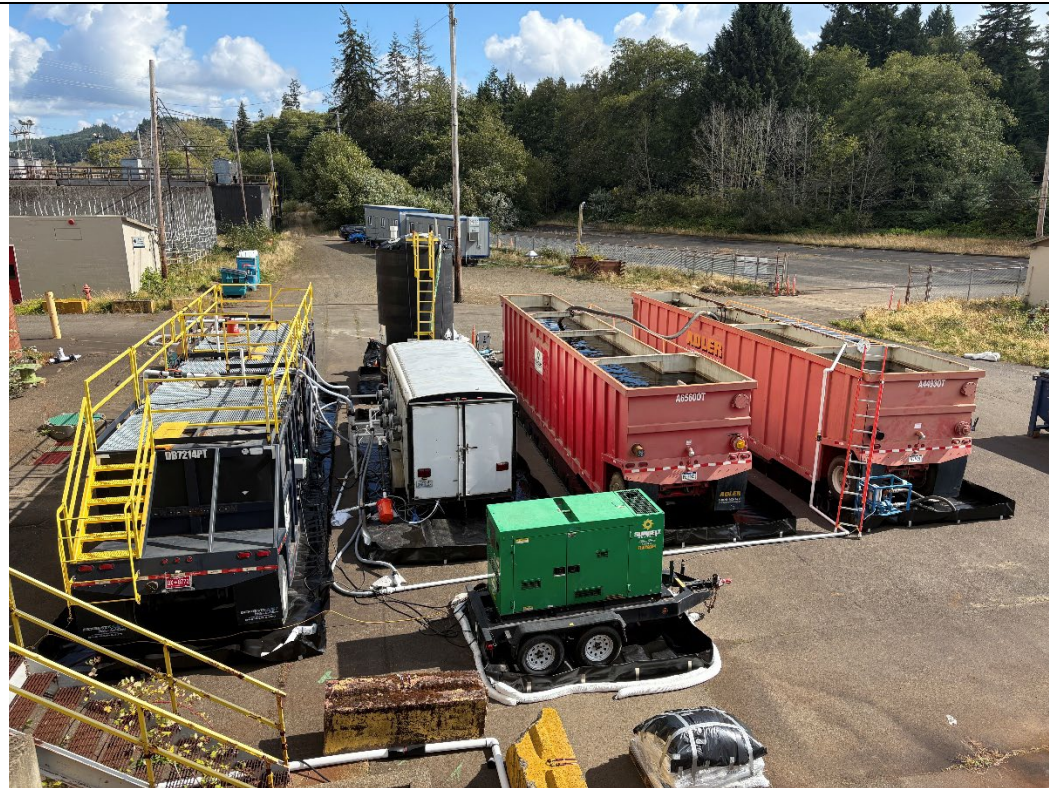
Another view of the fully constructed and operational waste treatment plant.
