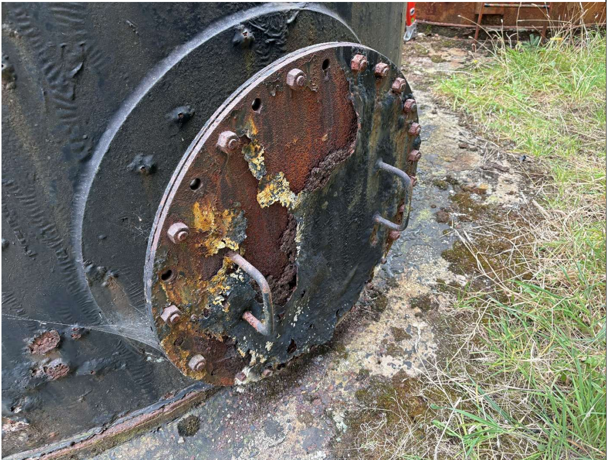
Heavily corroded and improperly sealed hatches (missing or absent bolts) on a tank full of corrosive chemicals.
