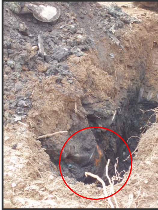
SITE: Alum Creek Bike Path Drum Site DATE: 11/8/2006 TIME: 0944 PHOTO NO: 3 DIRECTION: East PHOTOGRAPHER: Anne Busher SUBJECT: A shallow-buried 55-gallon drum in trench number2.
