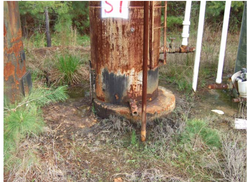
Site Name: Quality Petroleum, Inc.-Hoffman, et al. Project No.: E06614 Photo No.: 0212 Direction: W Contract No.: Date: 04/05/2008 Time: 9:41:00 AM Photographer/Witness: Sekerka, Robert/Johnson, Colin Description: E06614: Rust, corrosion and delaminated metal at base of S1.
