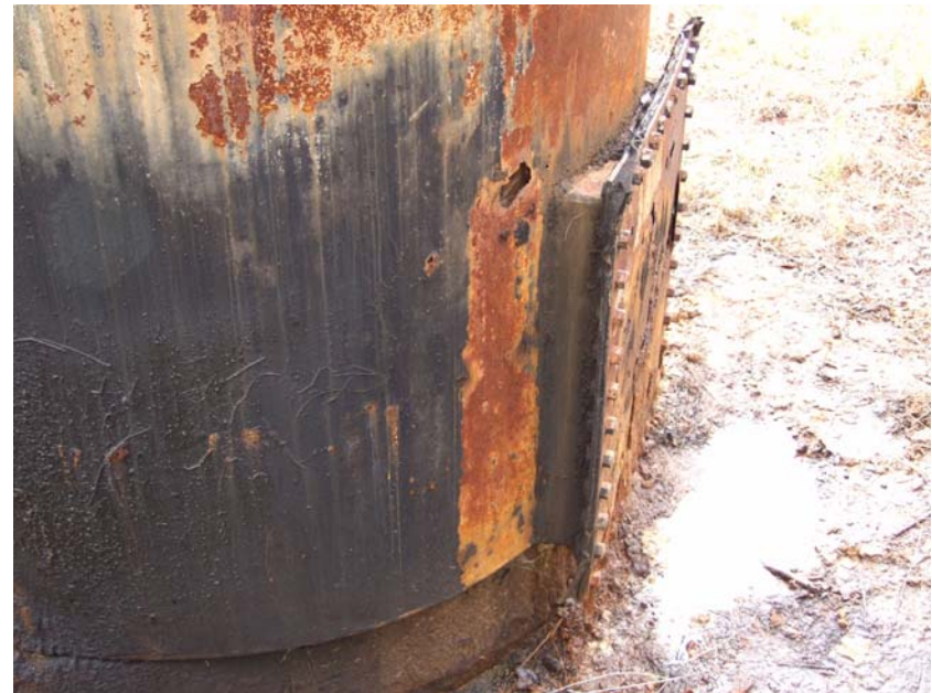
Site Name: Quality Petroleum, Inc.-Hoffman, et al. Project No.: E06614 Photo No.: 0214 Direction: Down Contract No.: Date: 04/05/2008 Time: 9:42:00 AM Photographer/Witness: Sekerka, Robert/Johnson, Colin Description: E06614: Rust, corrosion and delaminated metal on S1.
