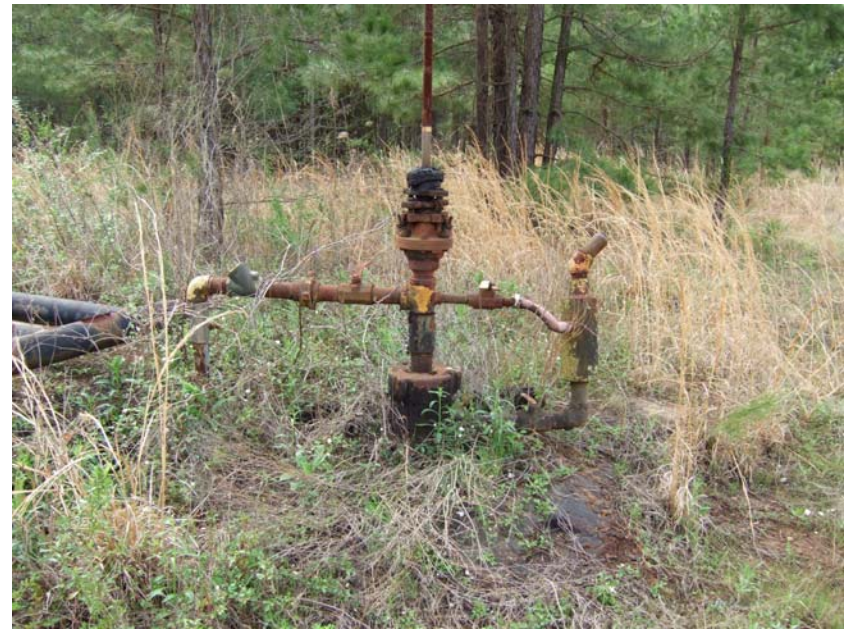
Site Name: Quality Petroleum, Inc.-Hoffman, et al. Project No.: E06614 Photo No.: 0218 Direction: NE Contract No. Date: 04/05/2008 Time: 9:48:00 AM Photographer/Witness: Sekerka, Robert/Johnson, Colin Description: E06614: Wellhead for SN 179621.
