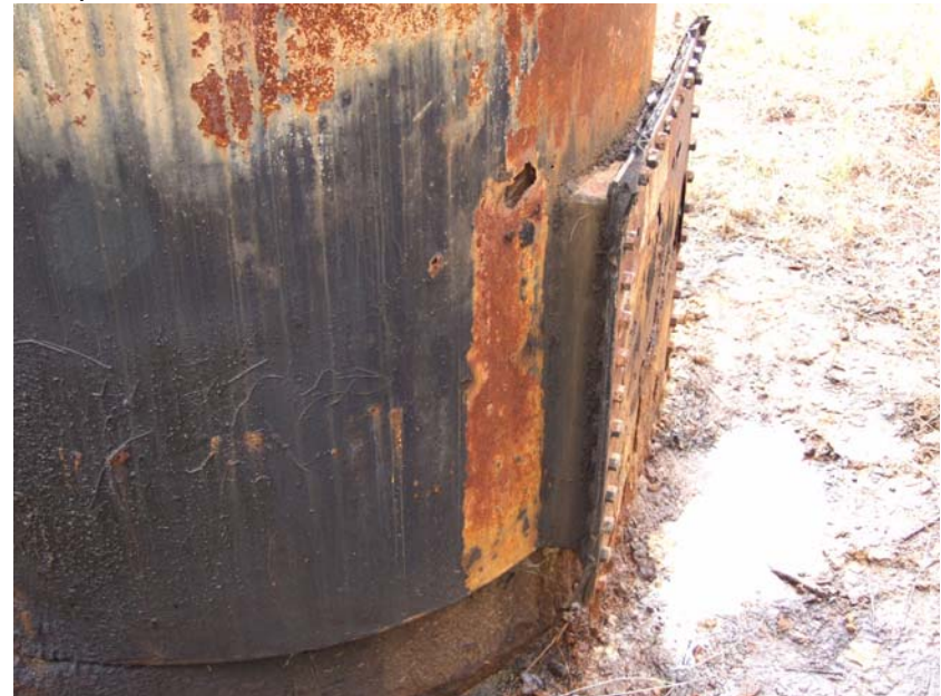
Site Name: Quality Petroleum, Inc.-Hoffman, et al. Project No.: E06614 Photo No.: 0214 Direction: Down Contract No.: Date: 04/05/2008 Time: 9:42:00 AM Photographer/Witness: Sekerka, Robert/Johnson, Colin Description: E06614: Rust, corrosion and delaminated metal on S1.
