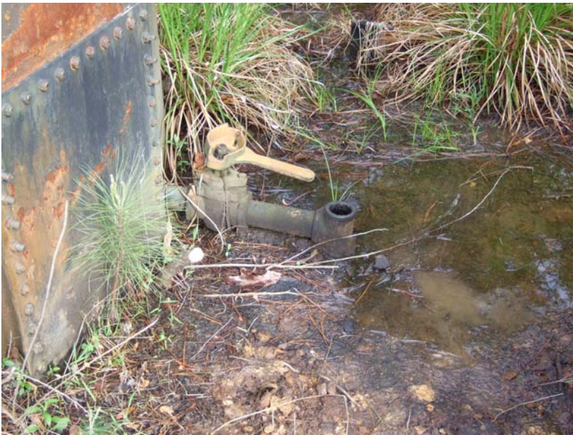
Site Name: Quality Petroleum, Inc.-Hoffman, et al. Project No.: E06614 Photo No.: 0209 Direction: Down Contract No.: Date: 04/05/2008 Time: 9:38:00 AM Photographer/Witness: Sekerka, Robert/Johnson, Colin Description: E06614: Oil saturated soil surrounding valve on AST2.
