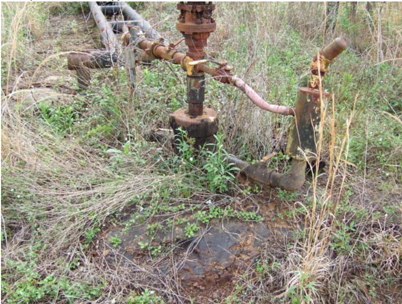
Site Name: Quality Petroleum, Inc.-Hoffman, et al. Project No.: E06614 Photo No.: 0219 Direction: Down Contract No. Date: 04/05/2008 Time: 9:49:00 AM Photographer/Witness: Sekerka, Robert/Johnson, Colin Description: E06614: Oil saturated soil around wellhead for SN 179621.
