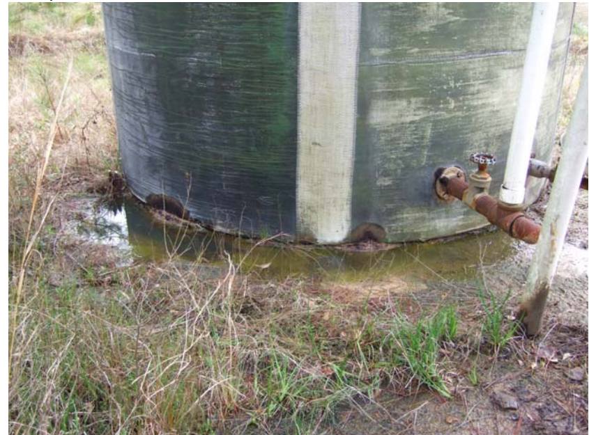
Site Name: Quality Petroleum, Inc.-Hoffman, et al. Project No.: E06614 Photo No.: 0216 Direction: Down Contract No.: Date: 04/05/2008 Time: 9:44:00 AM Photographer/Witness: Sekerka, Robert/Johnson, Colin Description: E06614: Oily liquid seeping through the chipped and peeling fiberglass at the base of AST3.
