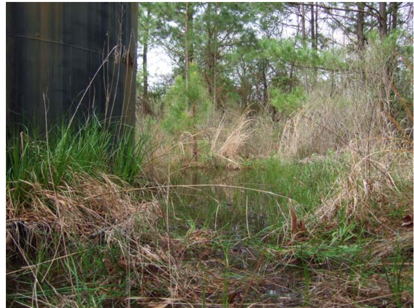
Site Name: Quality Petroleum, Inc.-Hoffman, et al. Project No.: E06614 Photo No.: 0206 Direction: SW Contract No. Date: 04/05/2008 Time: 9:36:00 AM Photographer/Witness: Sekerka, Robert/Johnson, Colin Description: E06614: Pooled water around AST1 Inside CONT1.
