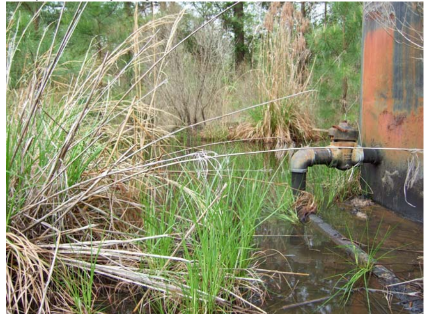
Site Name: Quality Petroleum, Inc.-Hoffman, et al. Project No.: E06614 Photo No.: 0204 Direction: SW Contract No.: Date: 04/05/2008 Time: 9:34:00 AM Photographer/Witness: Sekerka, Robert/Johnson, Colin Description: E06614: Oily sheen on pooled water southwest of AST1 in CONT1.
