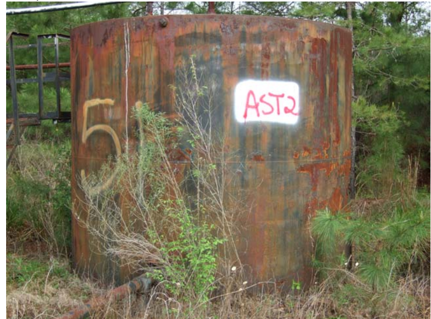
Site Name: Quality Petroleum, Inc.-Hoffman, et al. Project No.: E06614 Photo No.: 0208 Direction: W Contract No. Date: 04/05/2008 Time: 9:38:00 AM Photographer/Witness: Sekerka, Robert/Johnson, Colin Description: E06614: Label on AST2.
