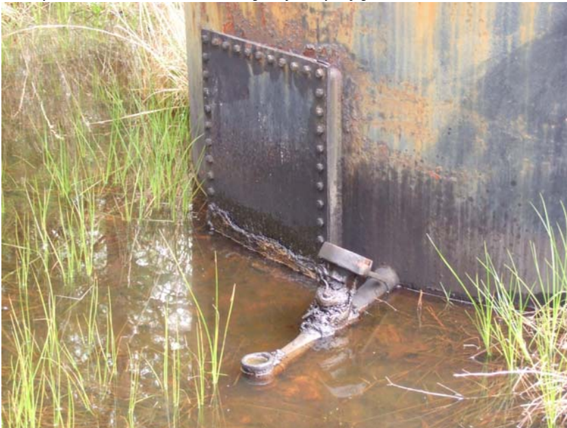
Site Name: Quality Petroleum, Inc.-Hoffman, et al. Project No.: E06614 Photo No.: 0207 Direction: NW Contract No. Date: 04/05/2008 Time: 9:37:00 AM Photographer/Witness: Sekerka, Robert/Johnson, Colin Description: E06614: Rust, corrosion and oily liquid seeping through the delaminated metal on the man way at the base AST1.
