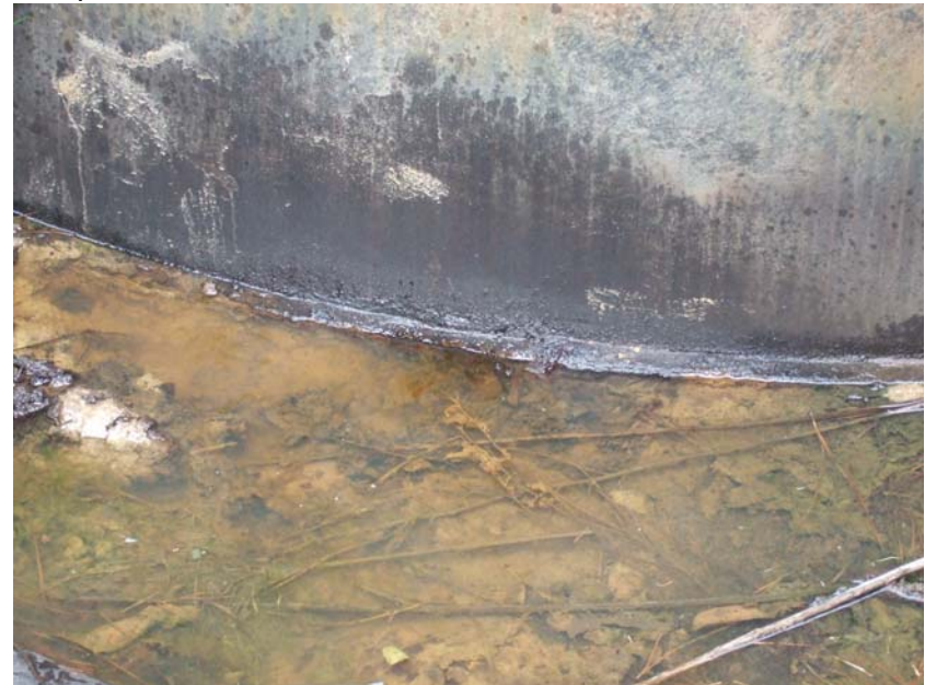
Site Name: Quality Petroleum, Inc.-Hoffman, et al. Project No.: E06614 Photo No.: 0220 Direction: Down Contract No. Date: 04/05/2008 Time: 10:12:00 A Photographer/Witness: Sekerka, Robert/Johnson, Colin Description: E06614: Pooled water around base of AST1.
