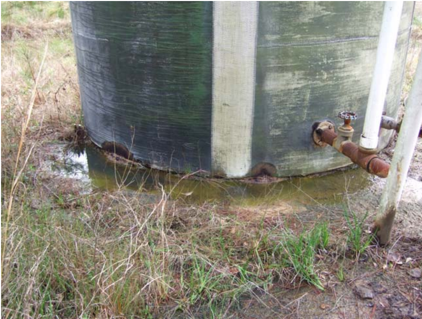
Site Name: Quality Petroleum, Inc.-Hoffman, et al. Project No.: E06614 Photo No.: 0216 Direction: Down Contract No.: Date: 04/05/2008 Time: 9:44:00 AM Photographer/Witness: Sekerka, Robert/Johnson, Colin Description: E06614: Oily liquid seeping through the chipped and peeling fiberglass at the base of AST3.
