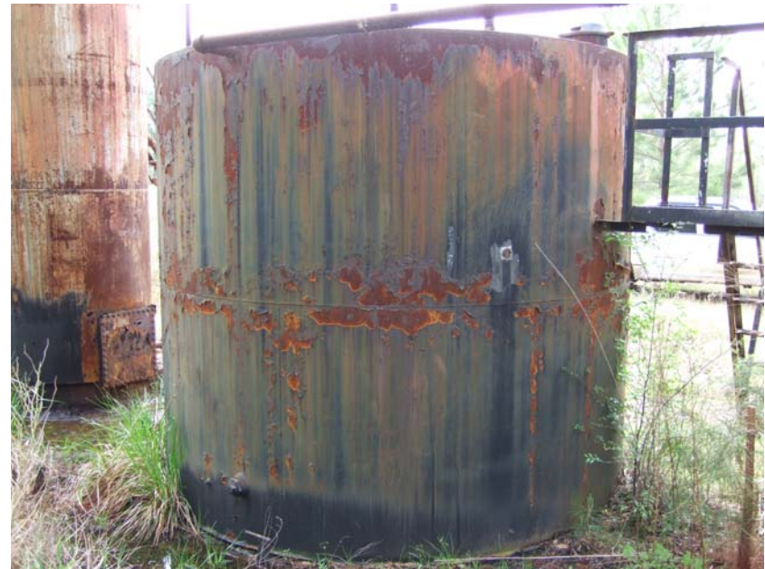
Site Name: Quality Petroleum, Inc.-Hoffman, et al. Project No.: E06614 Photo No.: 0210 Direction: E Contract No.: Date: 04/05/2008 Time: 9:39:00 AM Photographer/Witness: Sekerka, Robert/Johnson, Colin Description: E06614: Rust, corrosion and delaminated metal on AST2.
