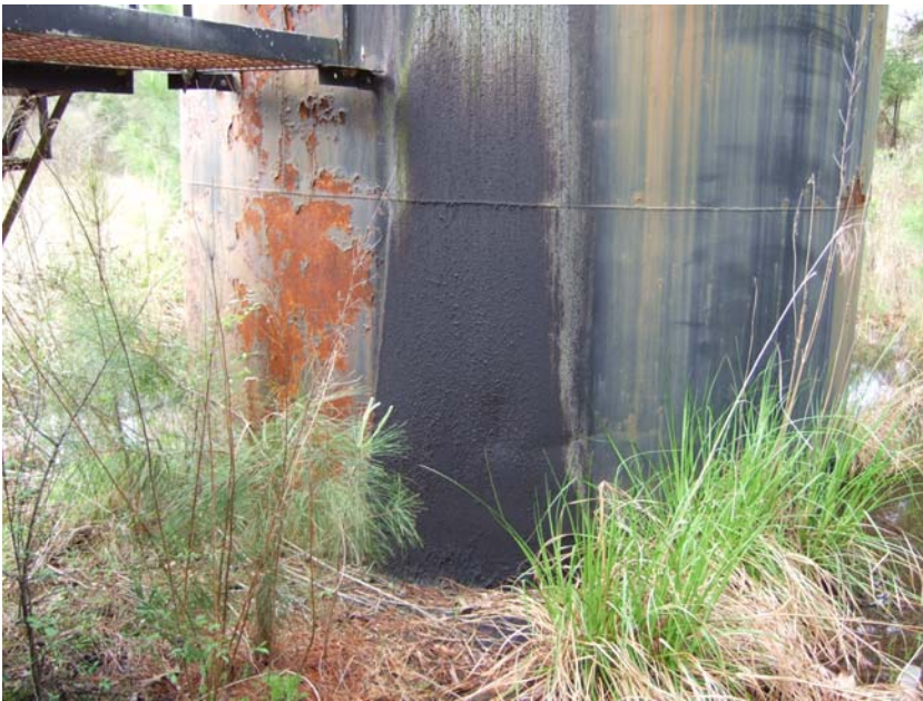
Site Name: Quality Petroleum, Inc.-Hoffman, et al. Project No.: E06614 Photo No.: 0205 Direction: SW Contract No. Date: 04/05/2008 Time: 9:35:00 AM Photographer/Witness: Sekerka, Robert/Johnson, Colin Description: E06614: Rust, corrosion and signs of prior oily seepage on AST1.
