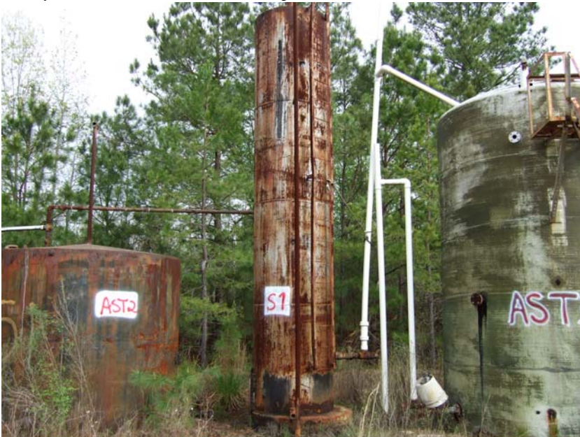
Site Name: Quality Petroleum, Inc.-Hoffman, et al. Project No.: E06614 Photo No.: 0211 Direction: W Contract No.: Date: 04/05/2008 Time: 9:40:00 AM Photographer/Witness: Sekerka, Robert/Johnson, Colin Description: E06614: Rust, corrosion and delaminated metal on S1.
