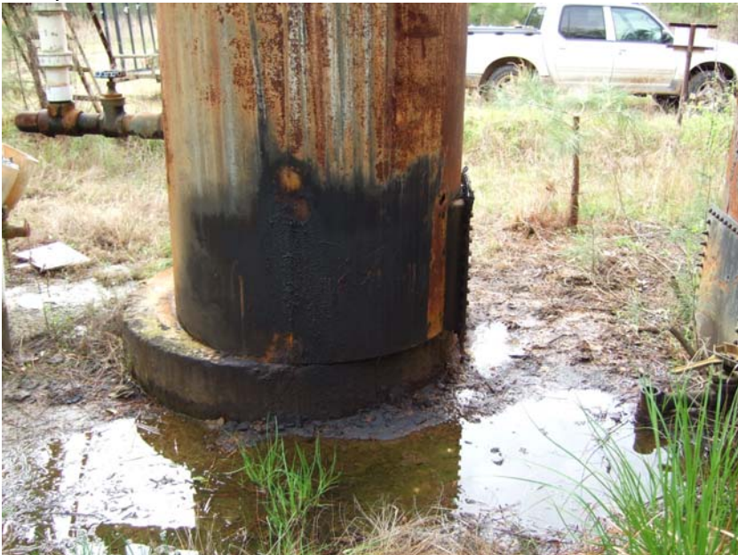
Site Name: Quality Petroleum, Inc.-Hoffman, et al. Project No.: E06614 Photo No.: 0213 Direction: E Contract No.: Date: 04/05/2008 Time: 9:41:00 AM Photographer/Witness: Sekerka, Robert/Johnson, Colin Description: E06614: Rust, corrosion and delaminated metal at base of S1 and evidence of prior oil release.
