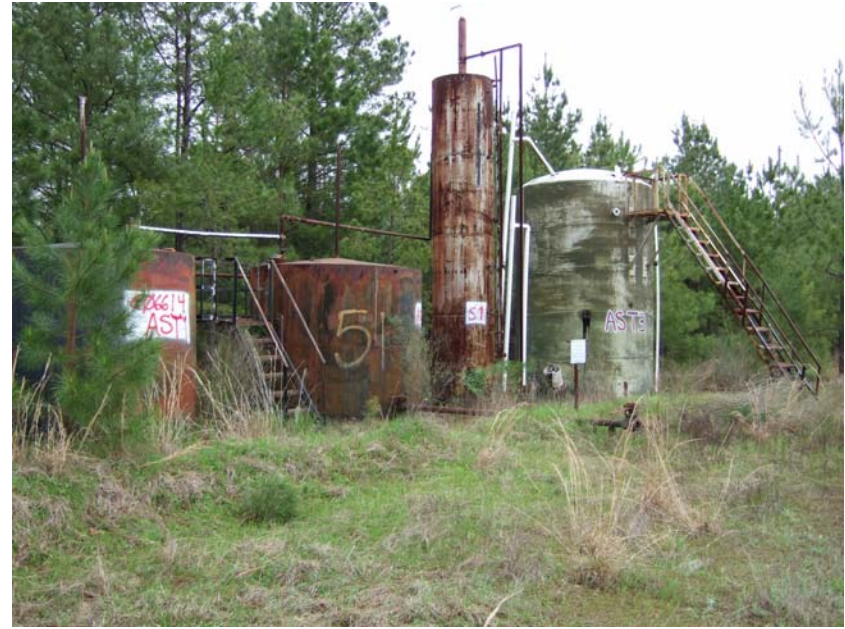
Site Name: Quality Petroleum, Inc.-Hoffman, et al. Project No.: E06614 Photo No.: 0201 Direction: NW Contract No. Date: 04/05/2008 Time: 9:28:00 AM Photographer/Witness: Sekerka, Robert/Johnson, Colin Description: E06614: AST1, AST2, AST3, and S1 in CONT1.
