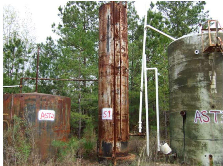
Site Name: Quality Petroleum, Inc.-Hoffman, et al. Project No.: E06614 Photo No.: 0211 Direction: W Contract No.: Date: 04/05/2008 Time: 9:40:00 AM Photographer/Witness: Sekerka, Robert/Johnson, Colin Description: E06614: Rust, corrosion and delaminated metal on S1.
