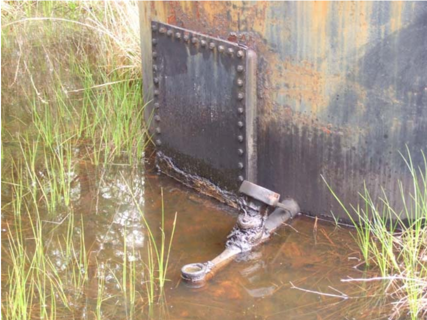
Site Name: Quality Petroleum, Inc.-Hoffman, et al. Project No.: E06614 Photo No.: 0207 Direction: NW Contract No. Date: 04/05/2008 Time: 9:37:00 AM Photographer/Witness: Sekerka, Robert/Johnson, Colin Description: E06614: Rust, corrosion and oily liquid seeping through the delaminated metal on the man way at the base AST1.
